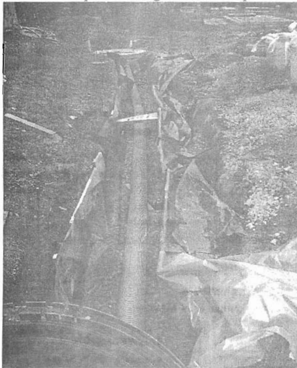
Plate (3) the filter drain during the fixation of the upper pipe (overflow pipe).
